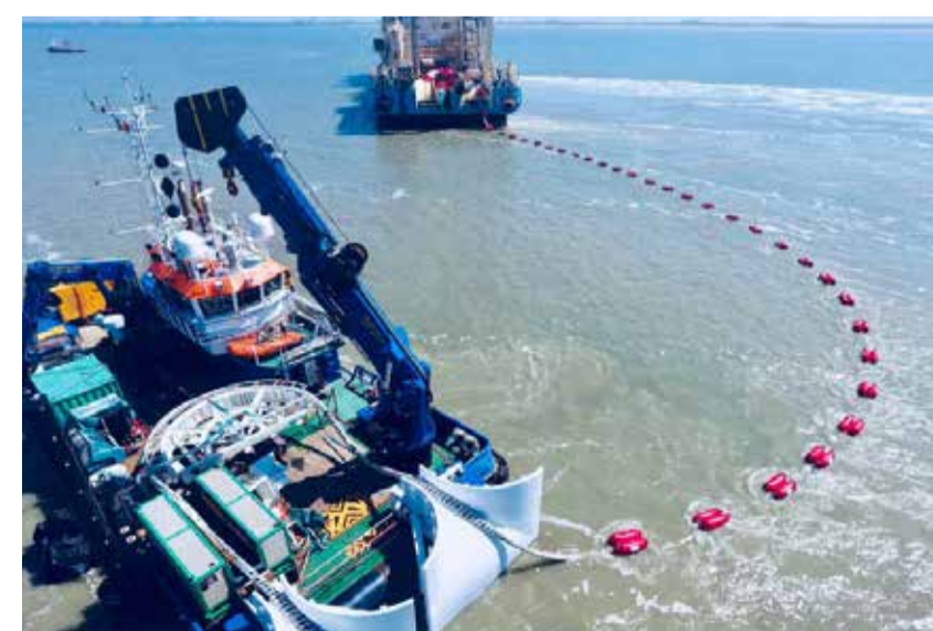
Marine cables will need to be installed in addition to underground cables.
