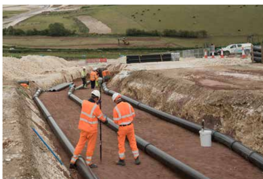
Cables will be installed 1-1.5 metres underground, as seen in the above image.
